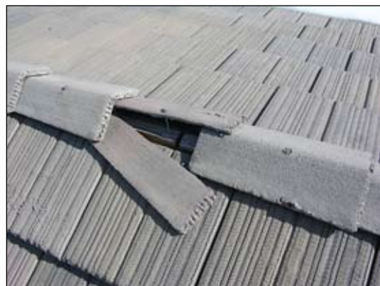
Figure 3. Displaced tiles allow ember entry.
